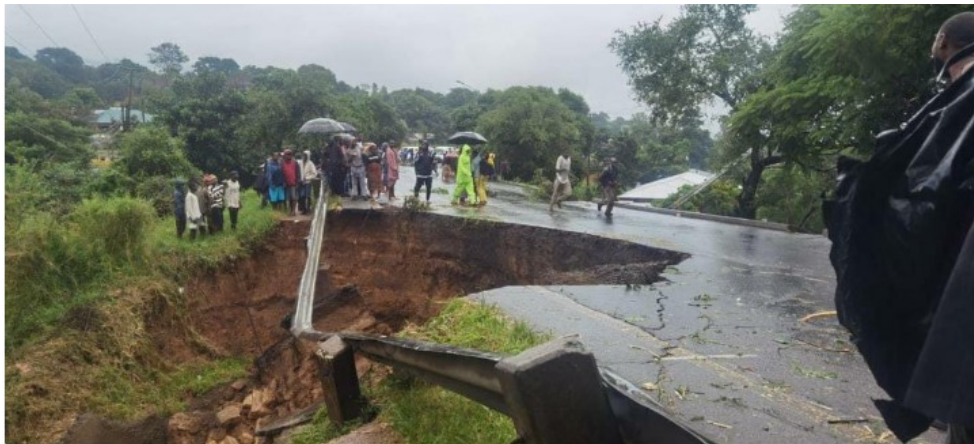
Figure 2. A Road Infrastructural Damage Caused by the Tropical Cyclone Freddy
